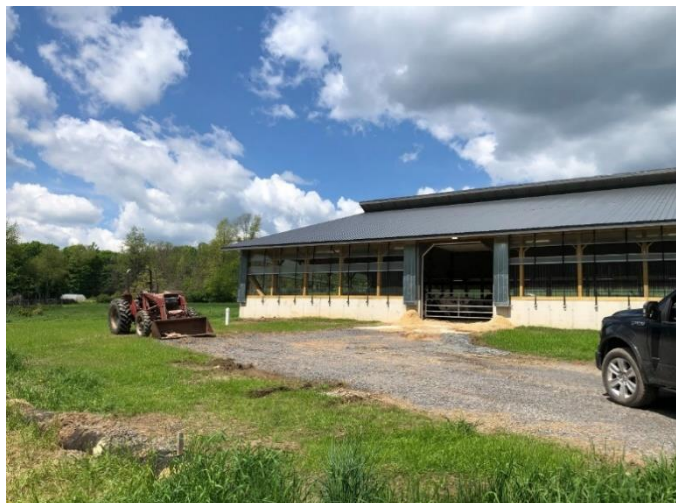
Luzerne County completion of The Lands at Hillside agricultural infrastructure and BMP upgrades.
