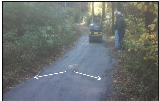
TSA can be successfully placed with small equipment for short sections of trail. Proper compaction at optimum moisture is crucial. Note the crown in the finished surface.
