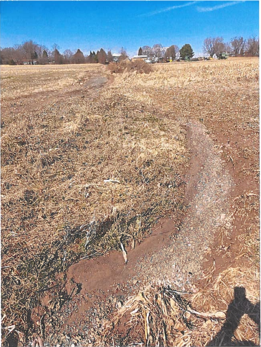
Access Road with Water bars and Stone lined Waterway
